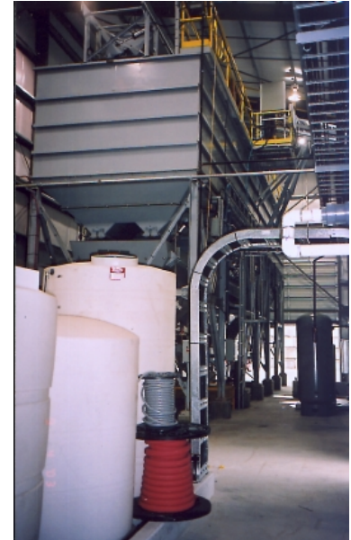
Interior of mixer plant
