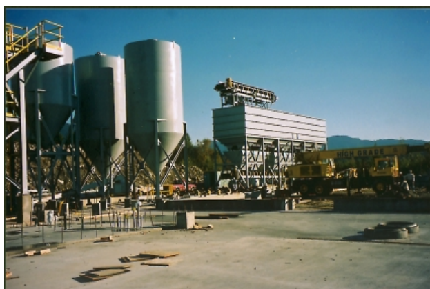
Installation of bins and silos
